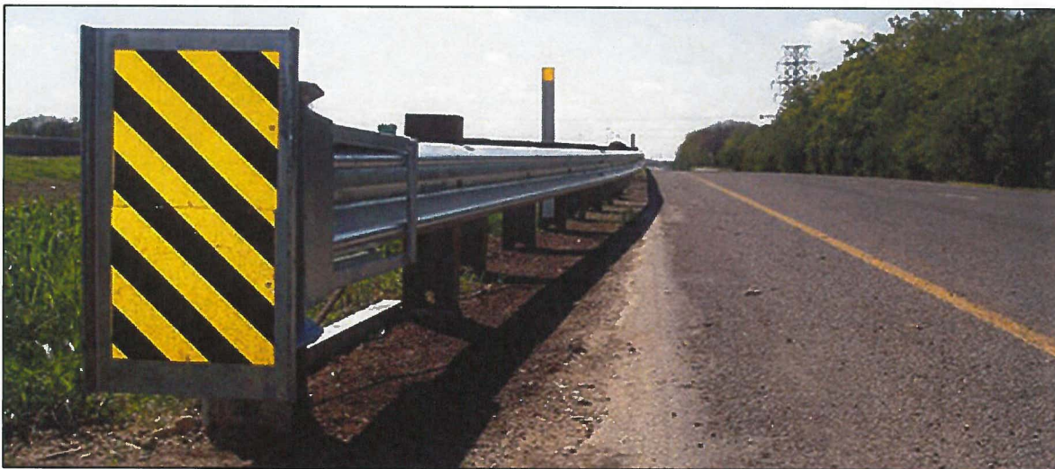
Example of Proper Guiderail End Treatment
