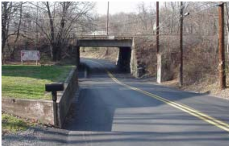
Photo of the view from westbound PA Route 849 approaching the Duncannon Subway
