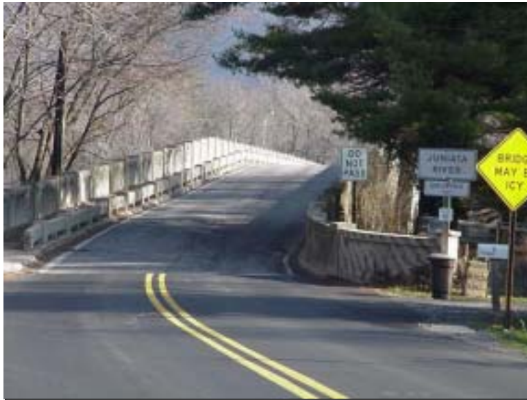
Photo of the view from eastbound PA Route 849 approaching the Juniata River Bridge
