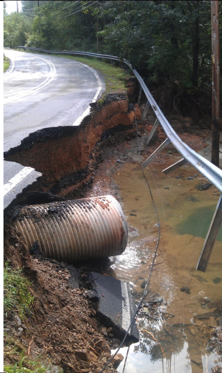
Figure 4.3.2-14 Flood impacts to Stoudt Road in South Hanover Township due to Tropical Storm Lee (September 2011) (South Hanover Township, 2011).
