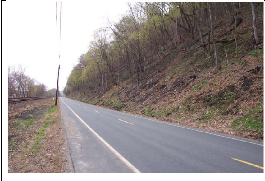
Figure 4.3.4-3 Known landslide hazard area along Route 147 north of Millersburg in Upper Paxton Township.
