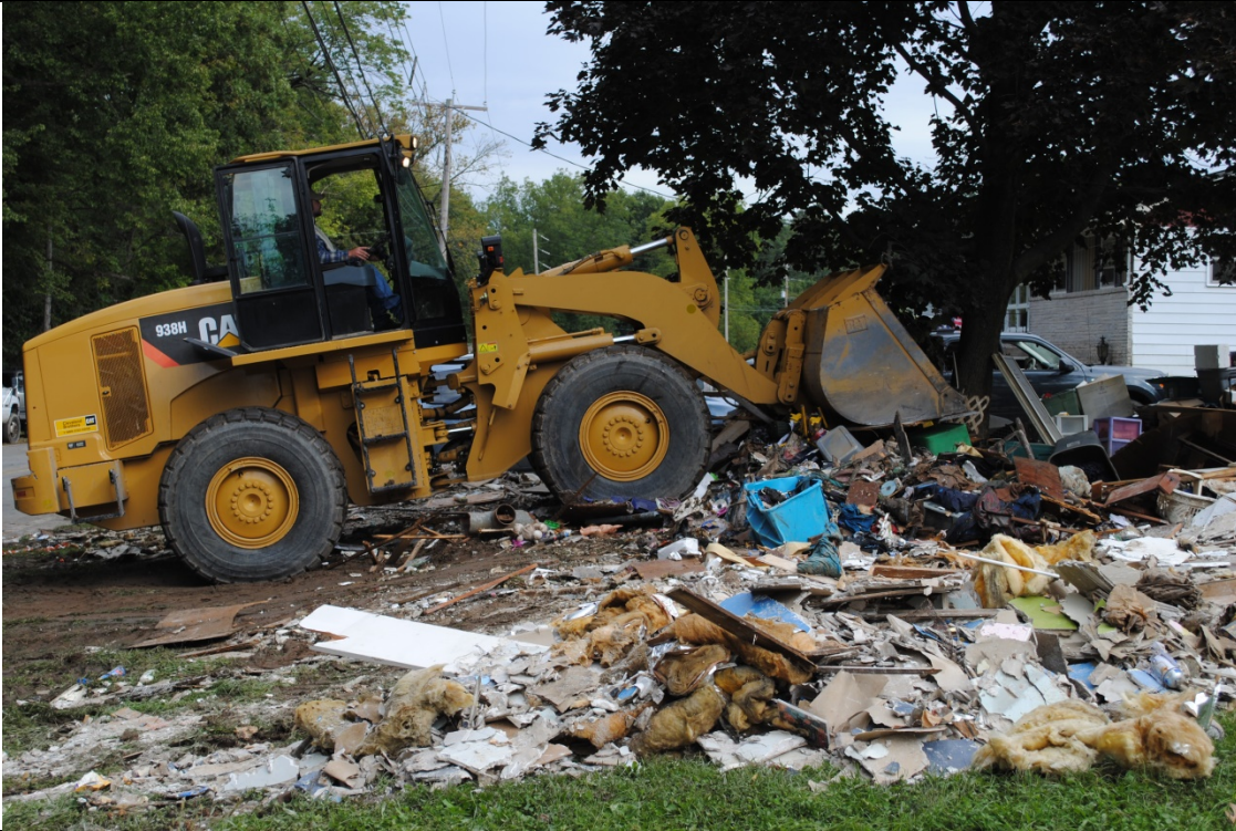
Figure 4.3.2-12 Cleaning up from flooding in Londonderry Township after Tropical Storm Lee (September 2011) (Londonderry Township, 2011).
