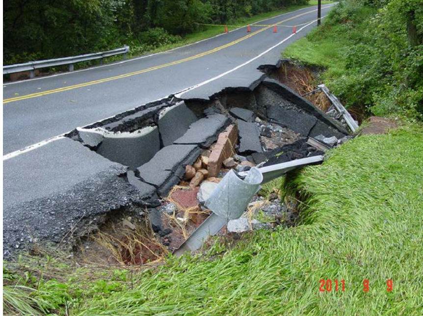
Figure 4.3.7-2 Sinkhole on Rosedale Avenue in Lower Swatara Township after Tropical Storm Lee.
